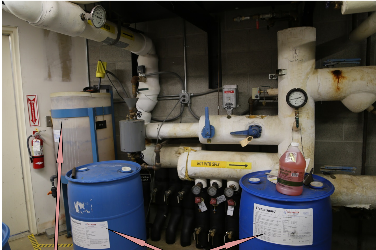
Glycol Feed Tank
